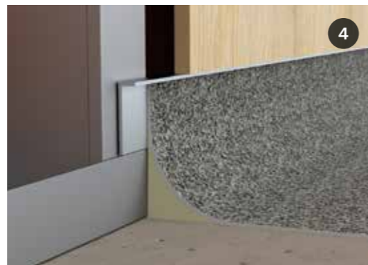
Raised vinyl floor
