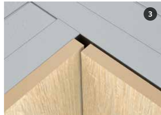
Open joint in internal corner
