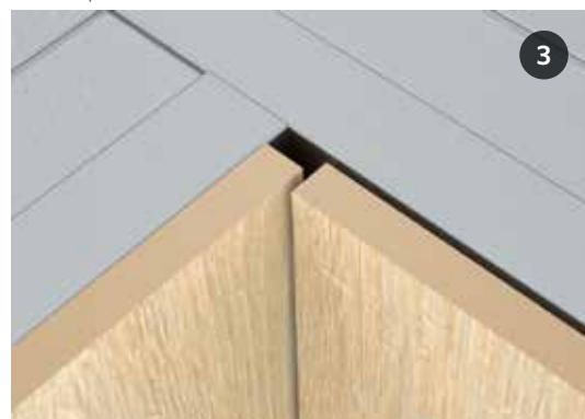
Open joint in internal corner
